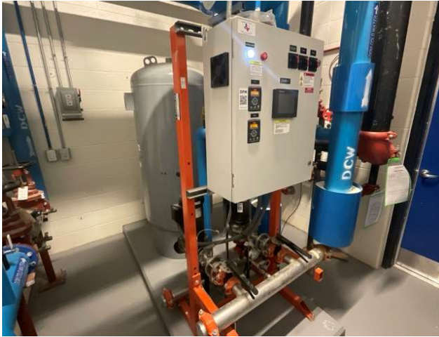
25 - DOMESTIC WATER PUMP STATION
