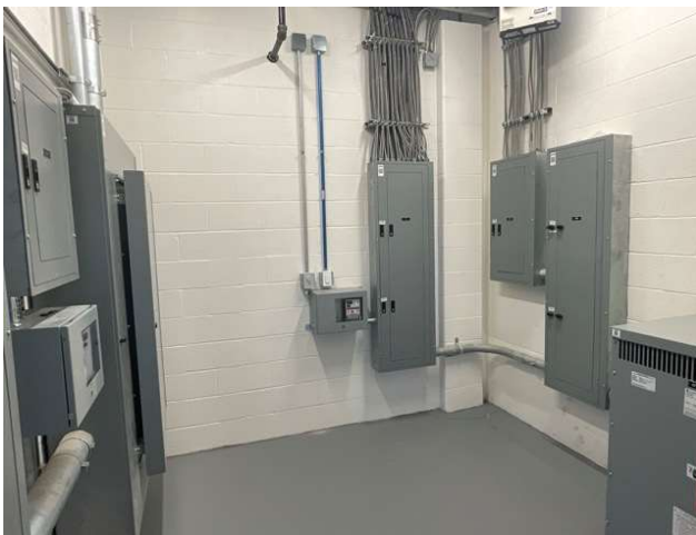
33 - ELECTRICAL ROOM (ADDITION)
