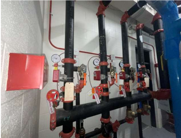
31 - FIRE SUPPRESSION SYSTEM
